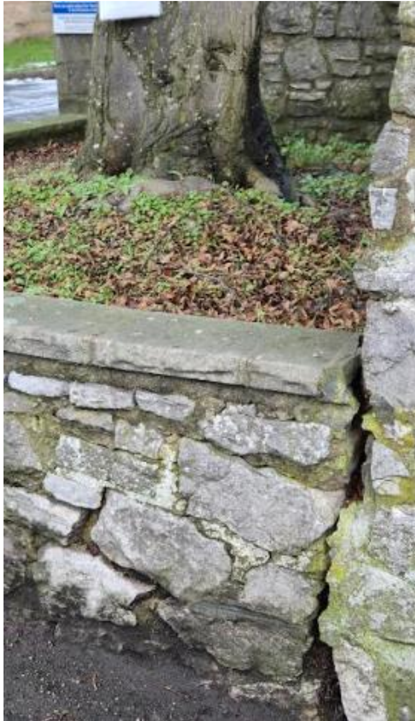
Plate 3. Showing the gap between the two walls adjacent to tree T1. This may be due to the walls not being tied into one another, or it may be due to displacement as asserted by the Objector. (this photograph was supplied by the Objector on 9th January 2026).
